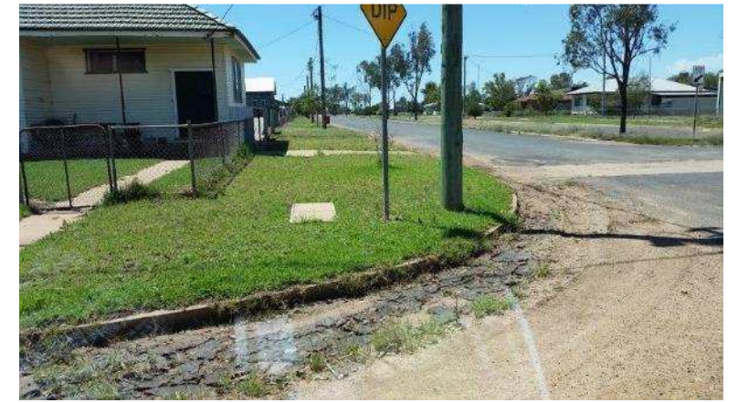
Cnr Clyde & Narromine Sts (evidence of standing water/drainage issues)
